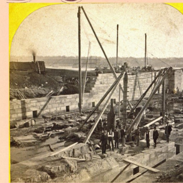
A view of workers on the Des Moines Rapids Canal, Keokuk, Iowa, ca. 1870 Courtesy of NYPL, Digital Collection, Photography Collection, Miriam and Ira D. Wallach Division of Art, Prints and Photographs
